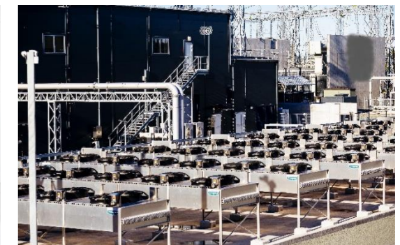
Plate 5.23 – Typical Outdoor Heat exchangers Image: ©GE
