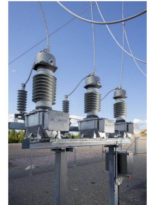
Plate 5.16 - Typical Voltage Transformer Image: ©ABB
