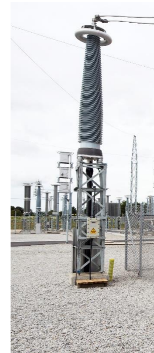
Plate 5.6 – Typical 400kV Cable Terminations Image: ©GE
