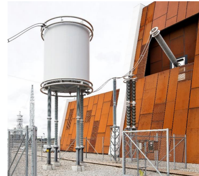
Plate 5.19 – Typical Phase reactors (outdoor) Image: ©GE
