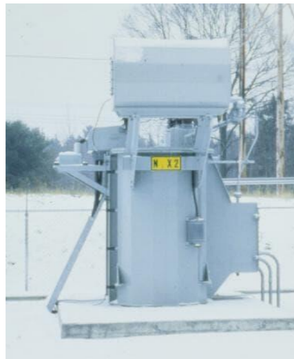
Plate 5.12 – Typical Auxiliary Power System Image: ©ABB
