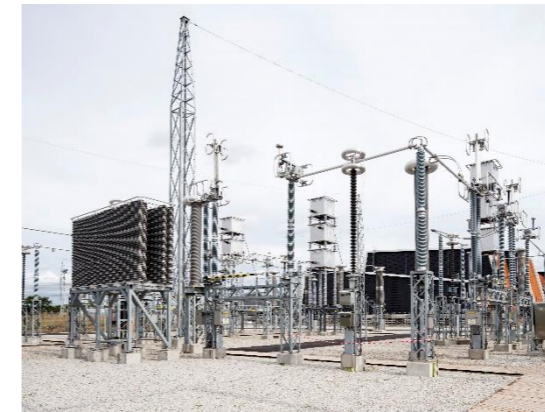
Plate 5.8 – Typical Lightning Masts Image: ©GE
