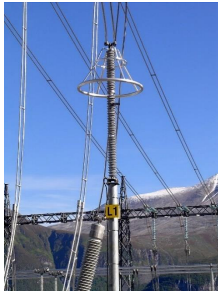
Plate 5.7 – Typical HV Surge Arresters Image: ©ABB
