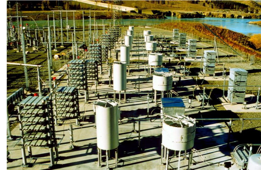
Plate 5.11 – Typical AC Switchyard Harmonic Filters Image: ©ABB
