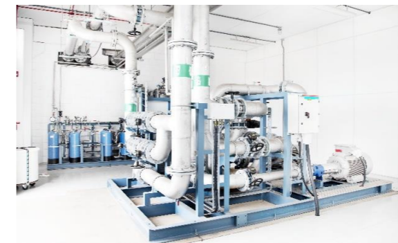
Plate 5.22 – Typical Water Pumping Station Image: ©ABB
