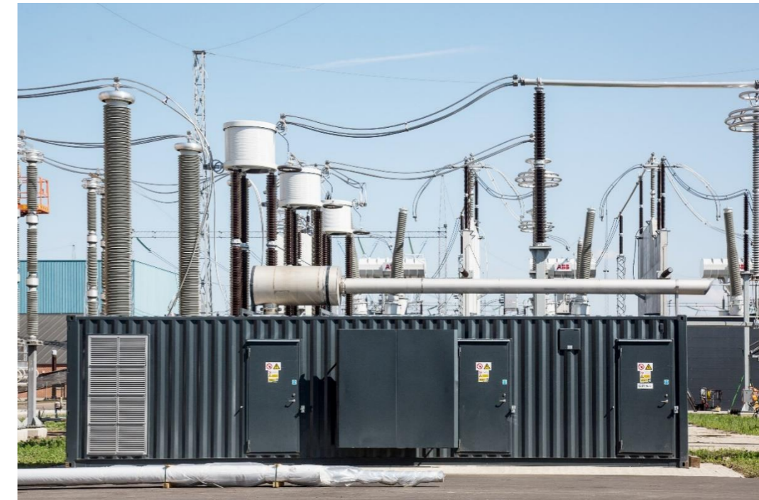
Plate 5.13 – Typical Diesel Generator Image: ©ABB
